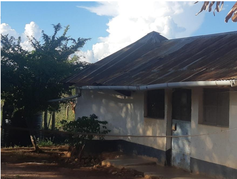
Figure 13: Example of how guttering is done to collect water from the roof to the tank
